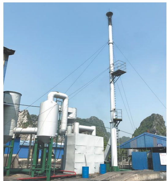
Exhaust gas treatment system
