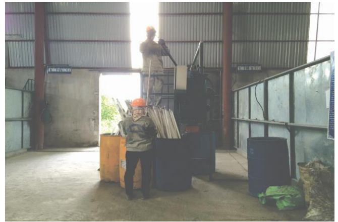
Mercury-contained bulbs treatment system
