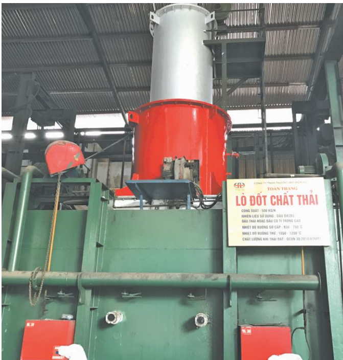
Burner system 500kg/h
