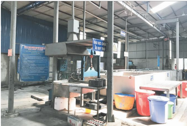
Discarded battery recycling system
